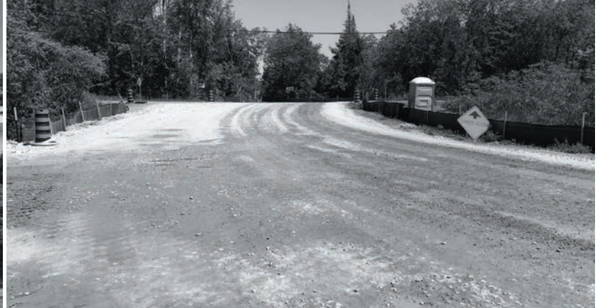
Much wider road to the hydro dam for heavy equipment during construction of expanded generating station.
