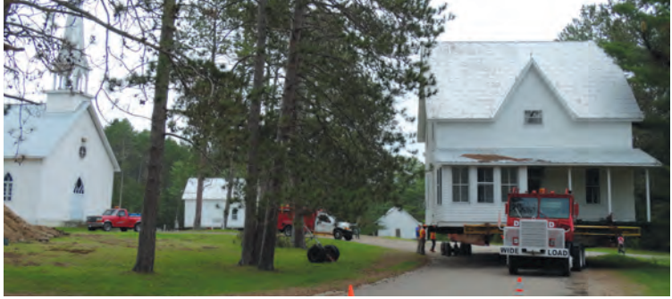
The 100 tonne rectory in position to be backed down the narrow road.
