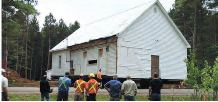
The Hall being pulled onto the prepared lot. "A lot of pies went through that window".
