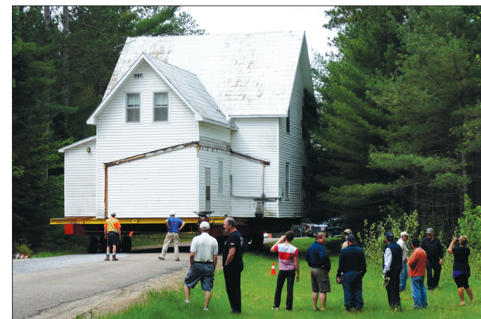
May 27, 2015 was an historic day for the village of Griffith. Many watched as Our Lady of the Holy Rosary Church rectory and hall were moved down the road. Story Pg. 14
