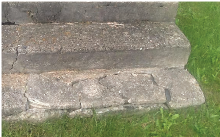
Broken steps at St. Gabriel the Archangel Church
