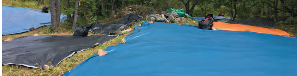
Clear anything that will keep tarps from lying flat and be prepared to leave them for 2 to 3 years.
