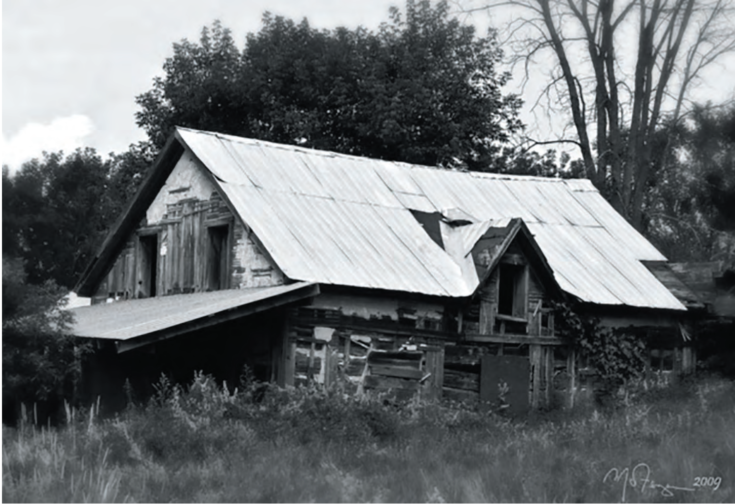
The long-abandoned Bill/Isabella Wilson home, the site of the First Wilson Post Office in Matawatchan but called Wilson. The house is situated on the MacPherson Farm in Matawatchan. For a lifetime, I have been convinced that this was the first Wilson Post Office site but in all my digging for the accompanying article, I could find no evidence that this was true. My grandfather, Walter Hutson was raised here by the Wilsons and told me many stories about those early times but since he died in 1967, much has become hazy. My impression may be correct but all who may have answered my questions have passed on. Pic by Mark Ferguson 2009
