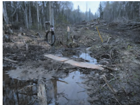
Bulldozing for transmission lines leaves a mess of rotting vegetation, inviting soil erosion...
