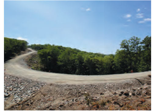
Blasted rock used to level new roads can become barriers to trails and old roads.
