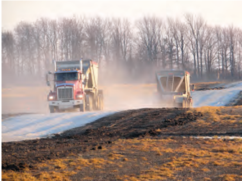
It takes a lot of gravel to make a road wide and strong enough for big turbine part trucking.
