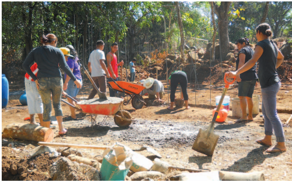
Everyone pitches in to dig a trench and pour a foundation. Helmets and steel toes not required.
