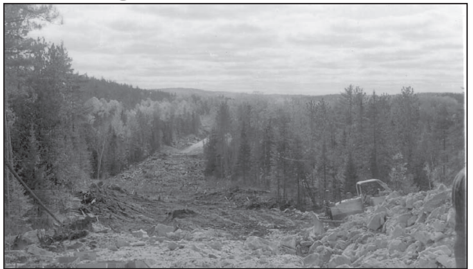
Clearing the bush for the Hydro dam at Black Donald. Photo: Francis McLelland
