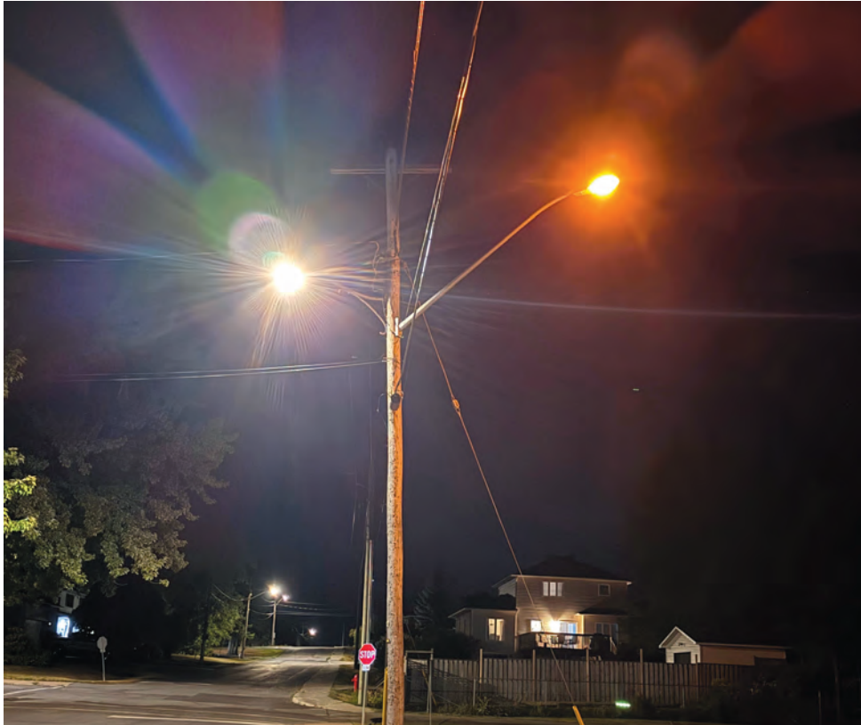
Colour difference between LED (left) and HPS (right) lights shows the colour and glare differences between new and old streetlights in this photo. The LED a blue-white hue is a newer light replaced by the Township for energy efficiency. The older style high pressure sodium (HPS) light is less efficient, but is a warm orange-white. (This particular HPS light wasn't replaced because it's on school property, not Township-owned property.) Photo: R. Scholes (CC-BY-NC 4.0)
