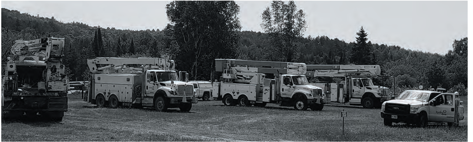
Hydro One trucks lined up along the Matawatchan Road near Griffith. Were we happy to see them! They fixed their lines in the area but need to come back to connect their lines to people's homes. The job still isn't complete.
