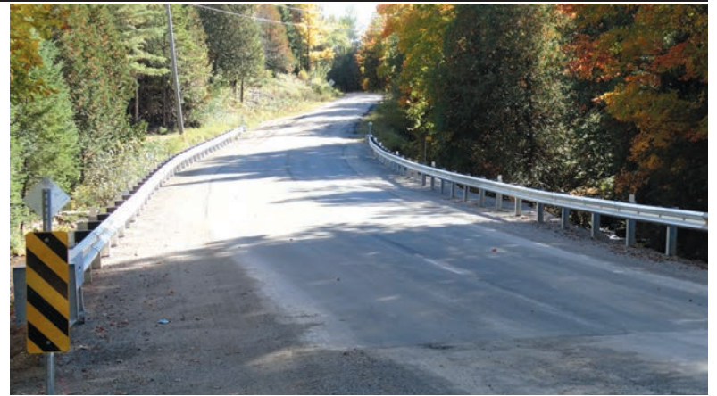
The work on the bridge over Colton Creek on Matawatchan Road is finally complete.
