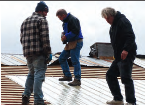
Peter Fischer, right, with Ben and Mike, two of the volunteers who worked for two days to replace the steel roof over the Bar section of the Hall in October. Thanks!
