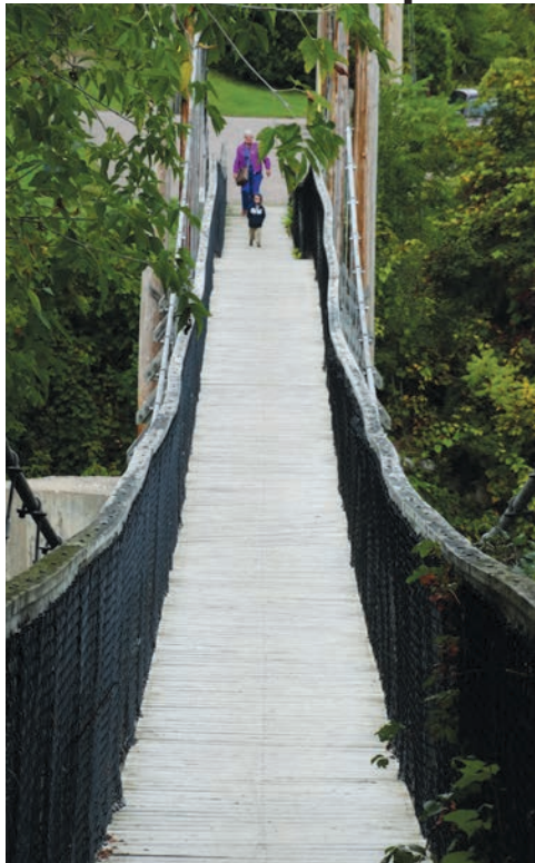
Swinging Bridge reopens at last, connected by new concrete stairs, built as part of the project.
