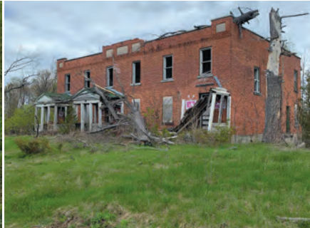
Row house where Hydro worker families lived. It had fallen into disrepair. Now they are privately owned and have now been demolished by their owners. Pic posted on Facebook by Craig Armstrong.
