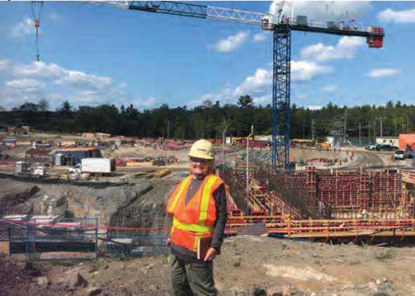
I was given a grand tour and treated like a VIP. Behind me is the new foundation. Pic taken from coffer dam. Rubble and rebar from 1917 Generation Station far in the background. The construction site is massive.
