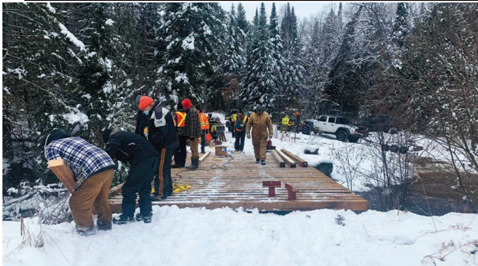
OFSC and OF4WD volunteers working together to re-deck a bridge on the Pencil Lake Trail. Supplied by: Peter Wood, President OF4WD
