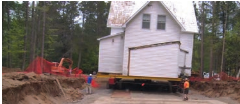
On May 27, 2015 the rector and hall were sold to Shawn Varrin and moved down the street by John LaCourse Carpentry. See the video at madawaskahighlander.ca/heritagerecordings
