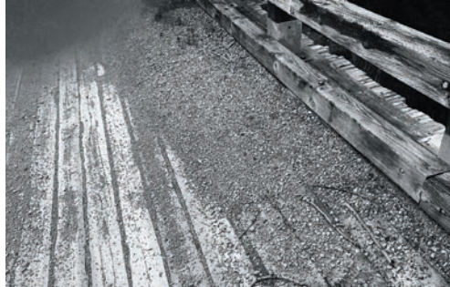
Gravel does not belong on the bridge. It is brought there by snowmobiles crossing when there is no snow there.
