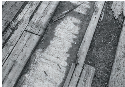
Wear and tear on the bridge on the K&P trail has made the surface unsafe for hikers and cyclists.
