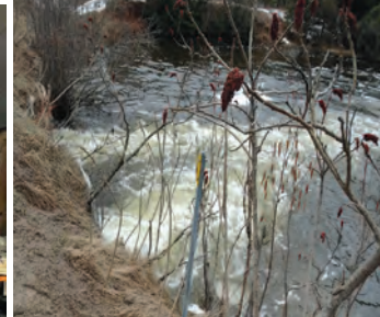
Water was only flowing properly through 2 of the 4 large culverts on Flying Club.
