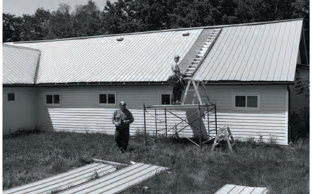
Jared Valliquette, who moved to Matawatchan recently, took on the job of replacing the rest of the steel on the Matawatchan Hall roof. He has taken over from Peter Fischer, who has retired and is working on his own projects now.
