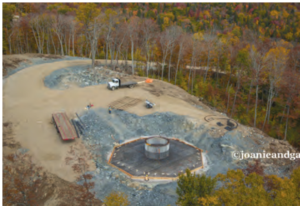
Windmill footings differ with each location. They must be buried and anchored to bedrock for stability. (Photo northernhoot.com Bow Lake Turbine Construction Northern Ontario ~Aerial Photography by Gary McGuffin.)
