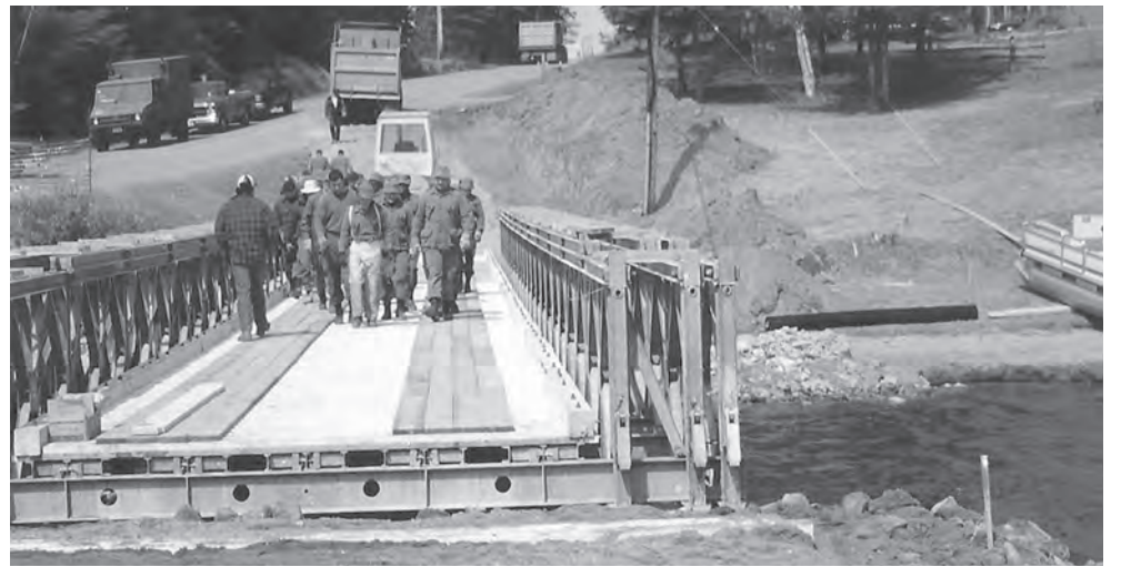
Royal Canadian Engineers on the almost completed Bailey Bridge over Lackie Creek near Camel Chute in 2003, after spring flooding took out the large culvert.
