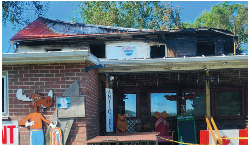
The original two storey 80-year-old Marble Lake Lodge burned on June 14 and cannot be saved, but most of the sections in front that were added later were spared or can be restored.
