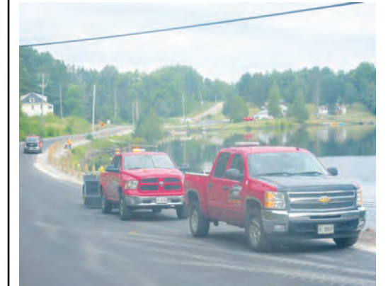
Resurfacing on Centennial Lake Road has just finished up. Enjoy the smooth ride.
