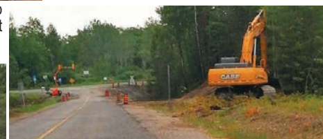
Centennial Lake Road is getting an overhaul, with better drainage and lines of sight.
