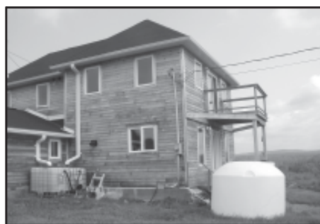
Water tank in yard. Drinking water system replaces worn out RO System. Rain water collection system is in the background.
